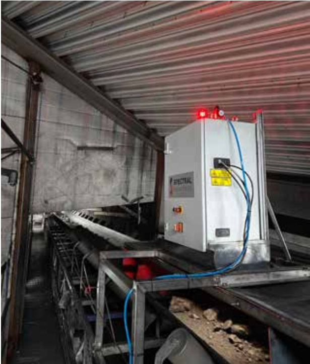
Figure 5 - Laser-based chemical sensors installed at the DINAMINE pilot sites provide real-time elemental measurements within ore streams, supporting process optimisation.
